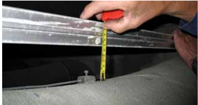
The reference tubes, made of conventional cast material (iron-nickel-chromium), had sagged 55–65 mm (2.2–2.6 in). Two of the reference tubes were replaced already after 1.5 years.
