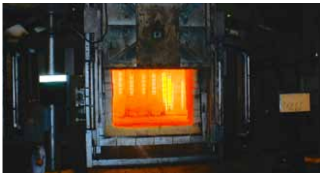
The rotary hearth furnace, 650 kW, with 56 Tubothal heating elements installed at Snecma.
