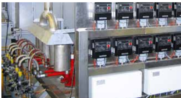
Each Ecothal 4-20 burner is individually controlled.
