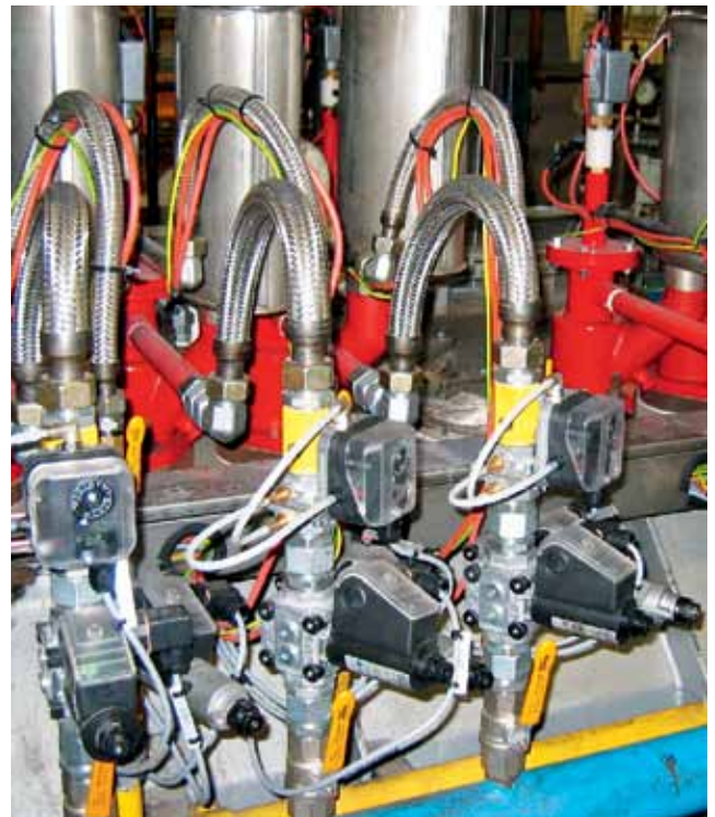
Ten Ecothal 4-20 burners serves the rebuilt oven.
